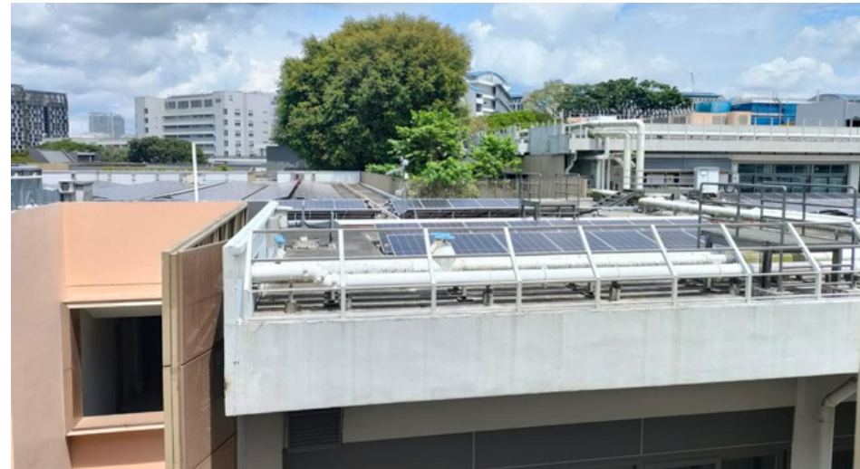
b) solar photovoltaic panels
